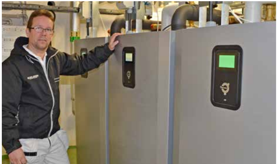
Anders Johansson at Thermia Mega heat pump
